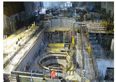
Cavern construction site at the Reißeck pumped storage power plant in Carinthia
