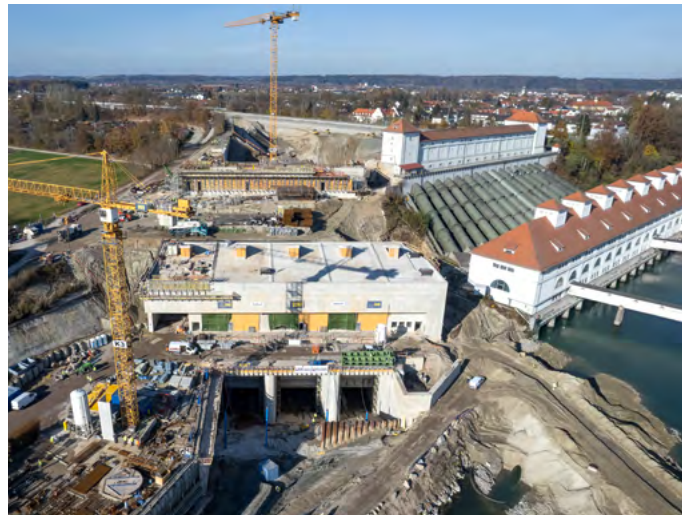
The new building for the Töging powerhouse (centre) with the existing installation to the right of the picture. The diversion channel in the background has already been emptied for the final work (stage of construction: September 2021).
