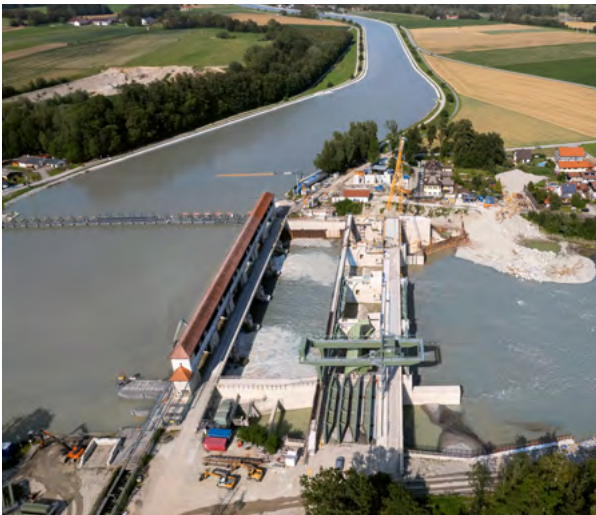
The existing Jettenbach weir (left) and the new construction (centre) looking onto the diversion channel (stage of construction: July 2021)
