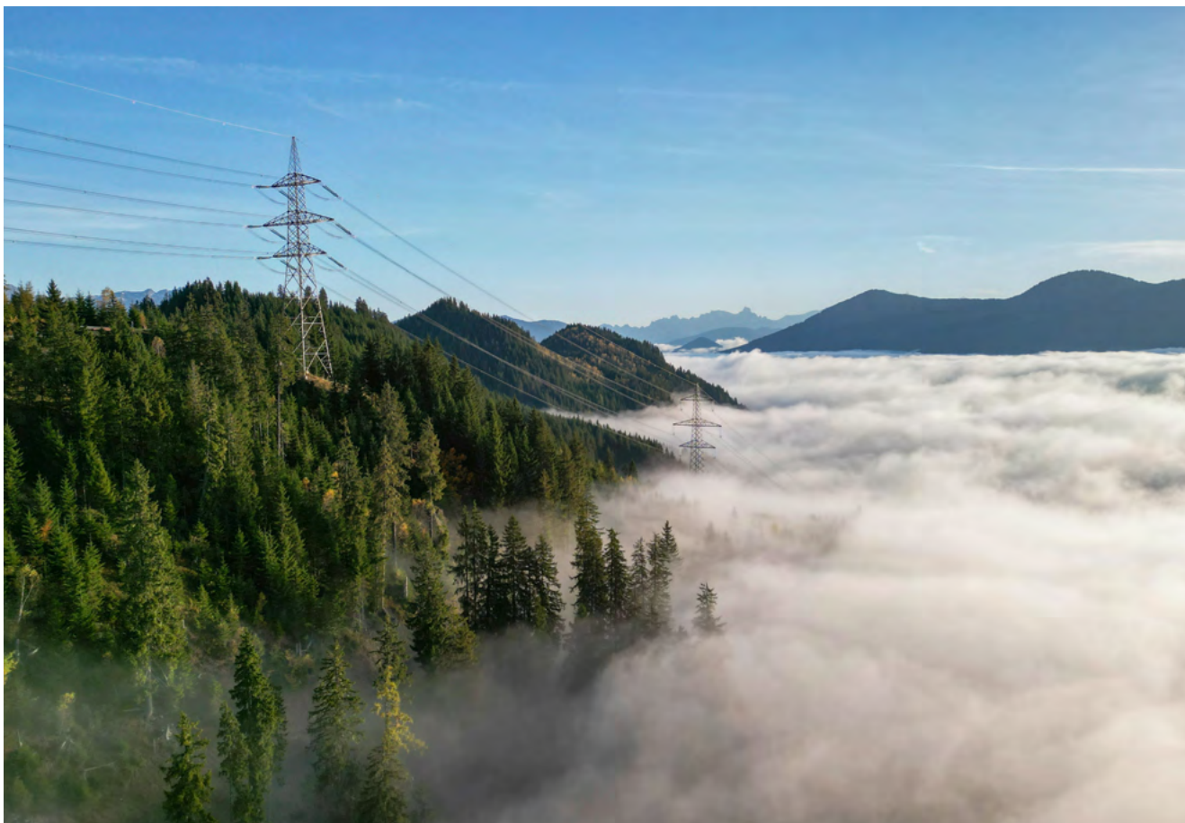
Image of the 380-kV Salzburg line. The Green Bond Committee proposes, reviews and evaluates projects to be financed with green funds.
