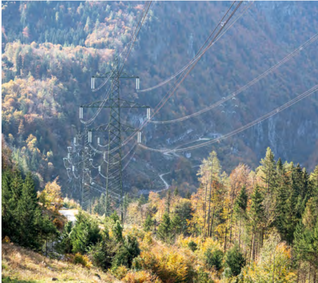
The new 380-kV Salzburg line has 449 pylons and 128 kilometres of transmission lines.
