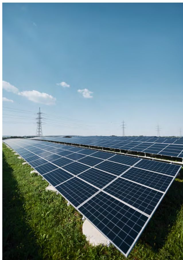
Open-field solar installation: the relevant revenue is recognised in the New renewables segment.
