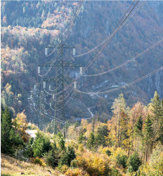
The new 380 kV Salzburg line has 449 pylons and 128 kilometres of transmission lines.
